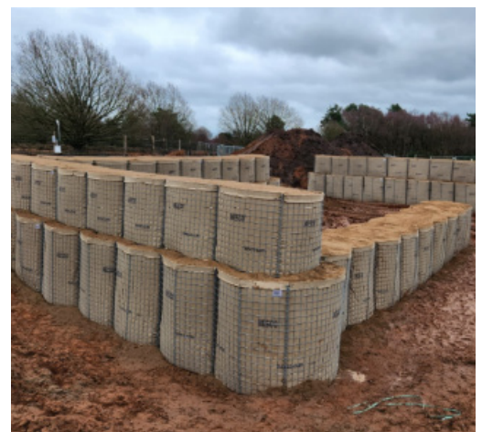
Image showing the HESCO Bastion blast protection installation which was used on-site in Nottinghamshire.
